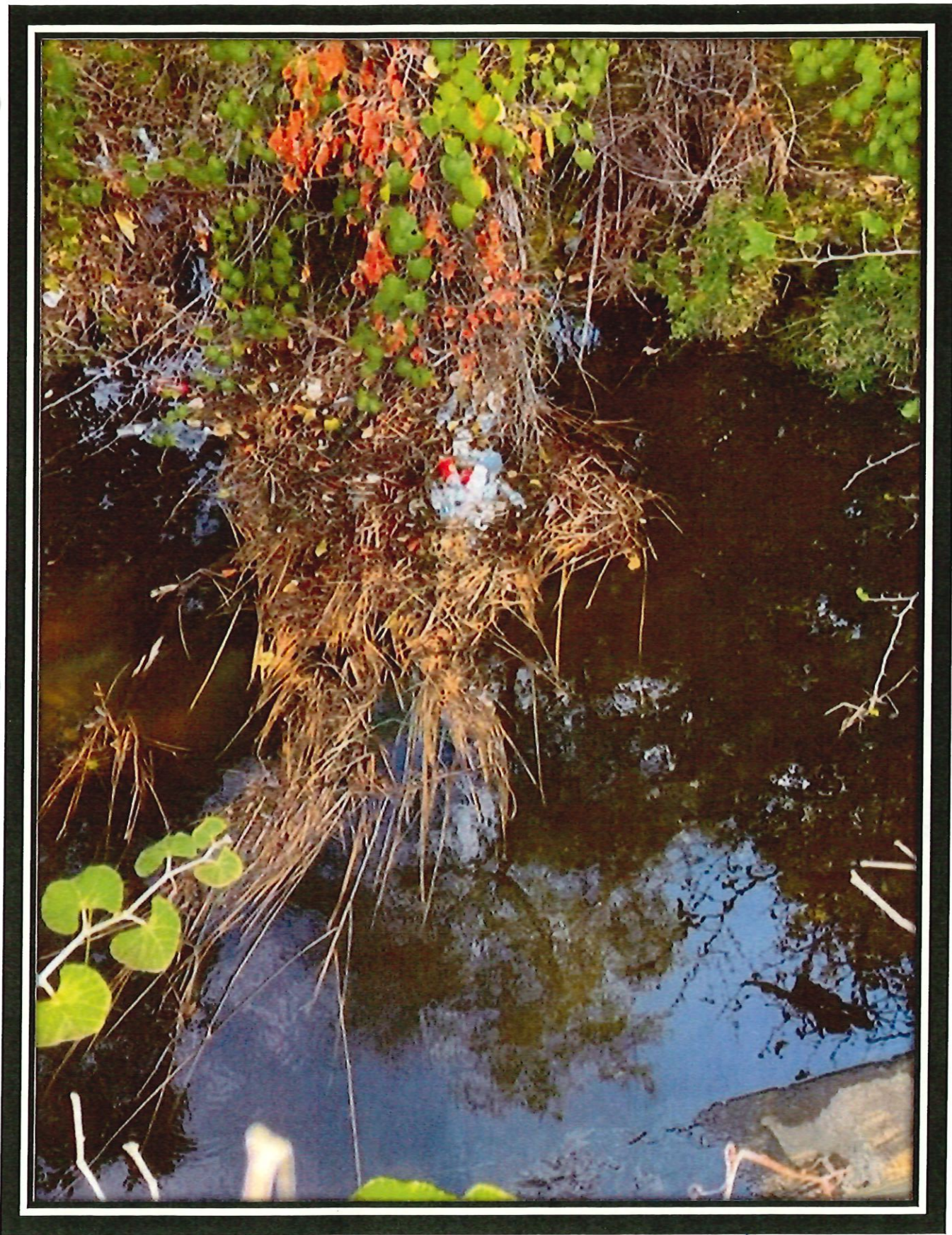
Stormwater Inspection of Outfall MC_005 on the far west side of campus on 09.19.2023. 20 KSA Note debris in stream which consists of mostly plastic bottles, some Styrofoam, and typical household trash. This stream is adjacent to the IM field where the trash bins are overflowing.
