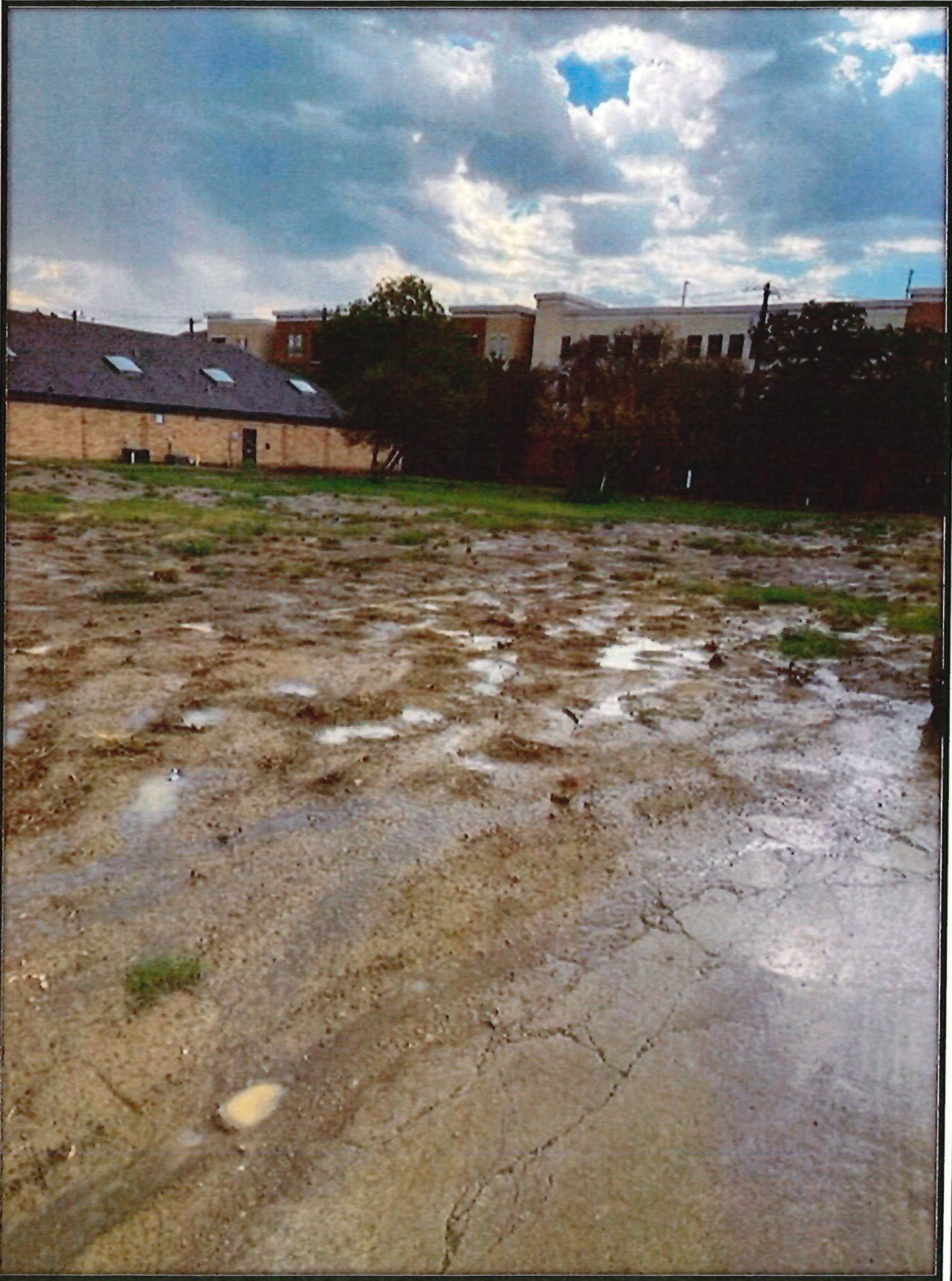
Stormwater inspection of Oak St. Hall property on 09.19 20 .2023. View is to the southeast.
