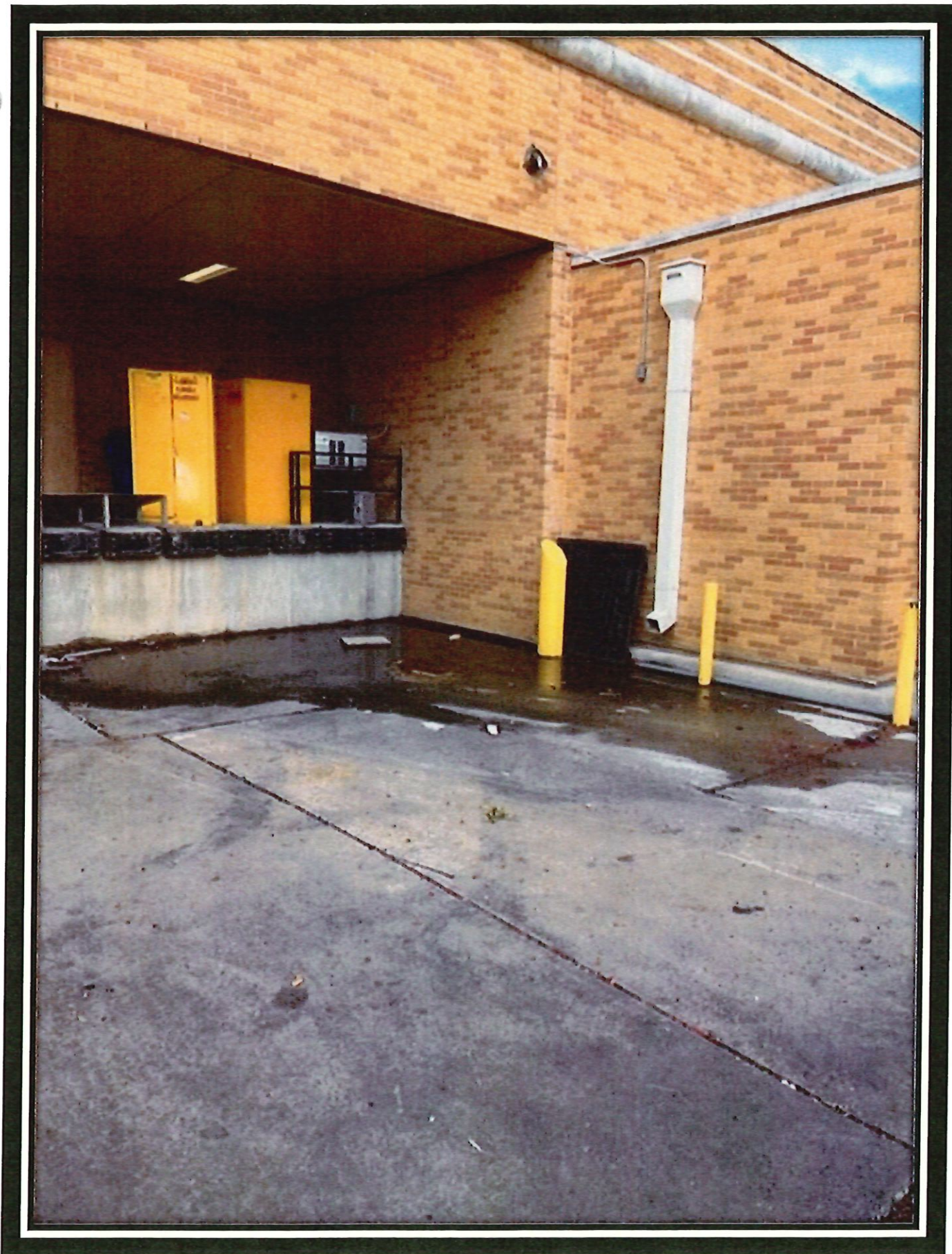
Stormwater Inspection of Science Research Building during renovation on 09.18. 20 2023. Loading dock area on north side of building with some standing stormwater and trash.
