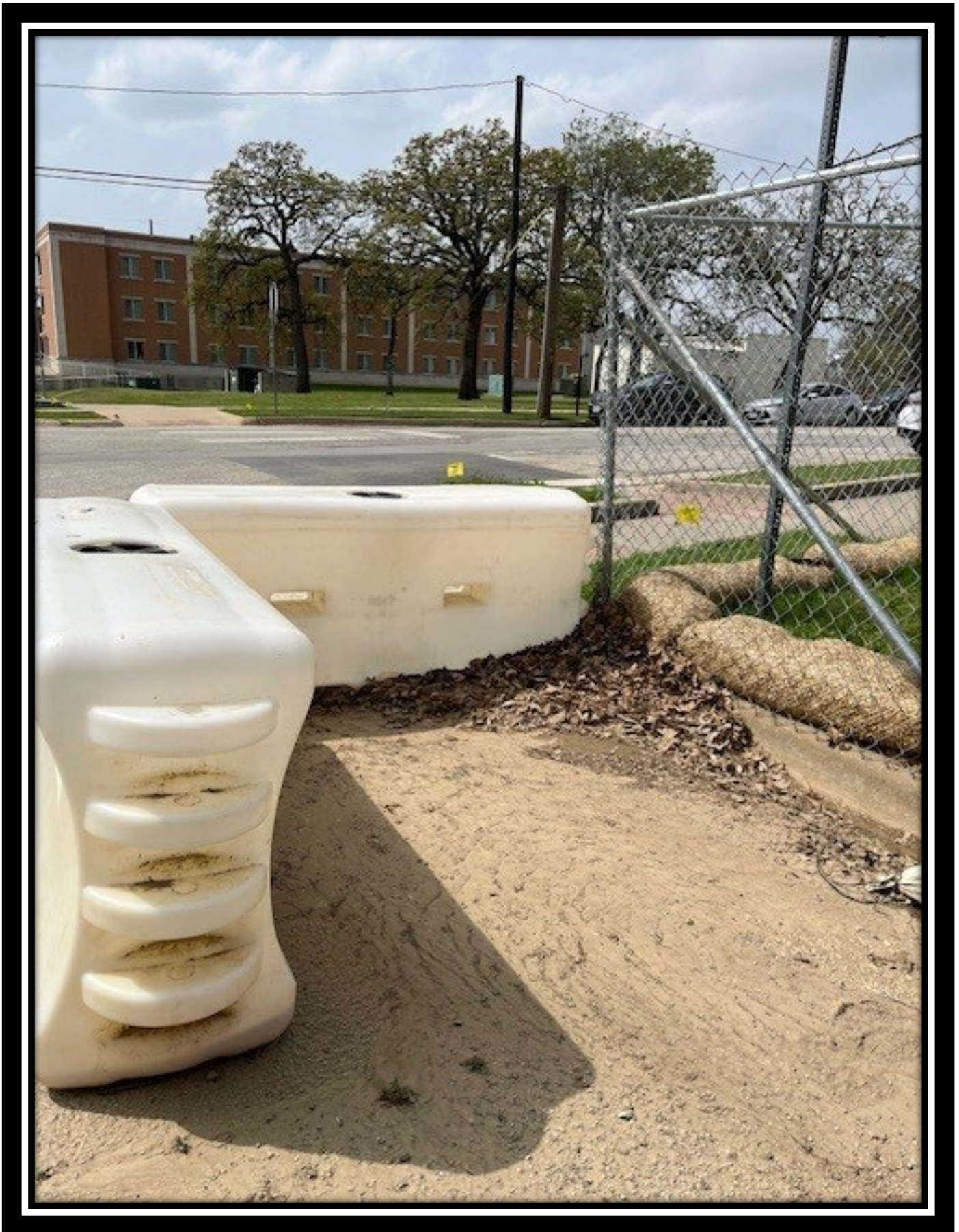
Soil and leaf litter build up at Avenue D and Sycamore Street during construction of the Science and Technology Building. (April 2025)
