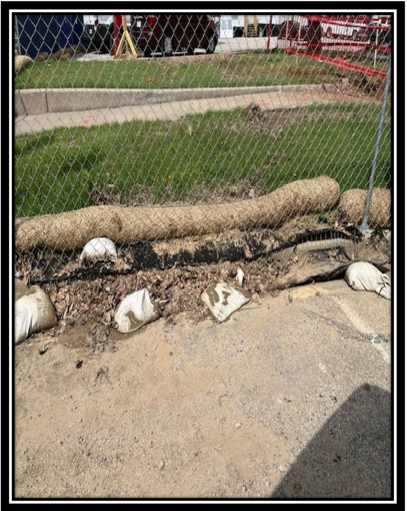
Stormwater curb inlet clogged Avenue D and Sycamore Street from runoff during the new Science and Technology Building construction project. (April 2025)
