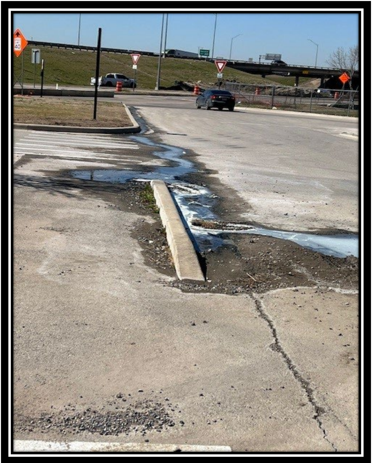
Sanitary sewer line break in Parking Lot 20 (February 2025). UNT Facilities repaired the broken sewer line in summer 2025.
