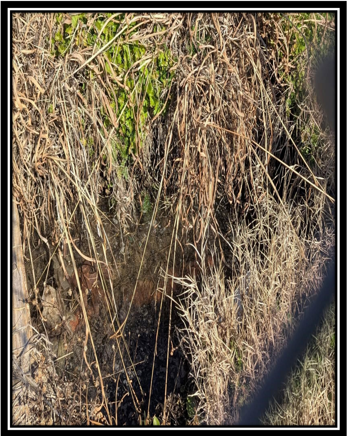
Broken water sprinkler on Traditions Band Practice field (February 2025).
