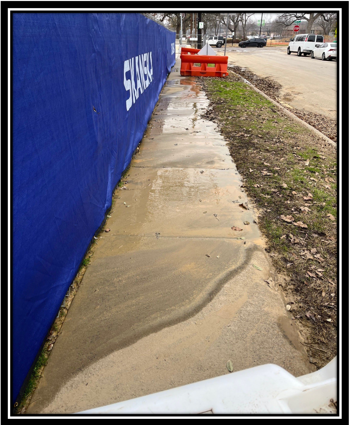
Dewatering the Science and Technology Building excavation pit. Precipitation in February contributed to the pit water. The construction contractor allowed it to run off onto the sidewalk and into the street. The sidewalk was cleaned by the construction contractor, and the pit water was eventually allowed it to infiltrate into the ground surface on-site. (February 2025)
